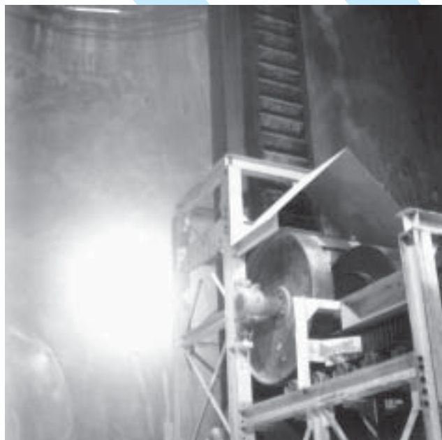
Deflection wheels under the city of Chicago used to excavate storm sewers.
