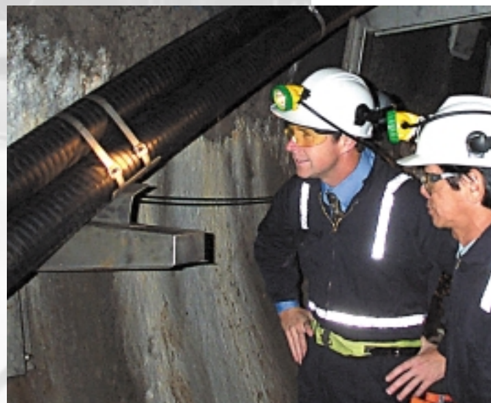
Underground cable in New Zealand is secured with fireproof BAND-IT stainless steel clamps
